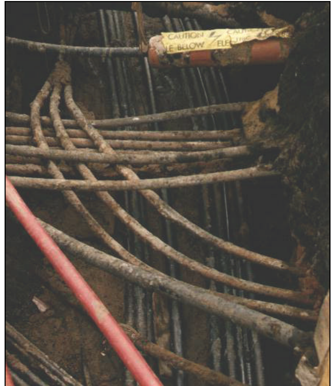
Figure 9: Congested trench in brown field site, with double circuit of 132kV lean cables passing underneath
