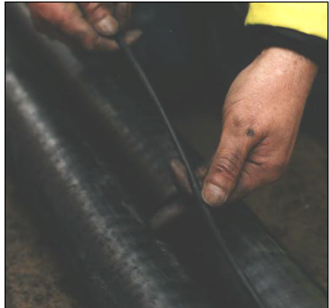
Figure 10: Inserting optical fibre temperature monitoring cable in centre of trefoil group of 132kV lean cables
