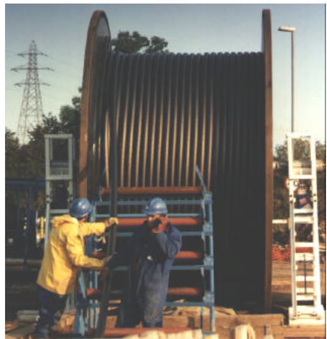
Figure 7: Pulling-in a 1.5km length of 132kV 630mm 2 lean cable, the winch for the wire bond is on the left hand side
