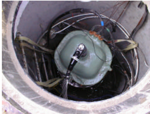
Figure 2 Fiberglass transformer installed in a regular sewer pipe showing connections and monitoring wiring.
