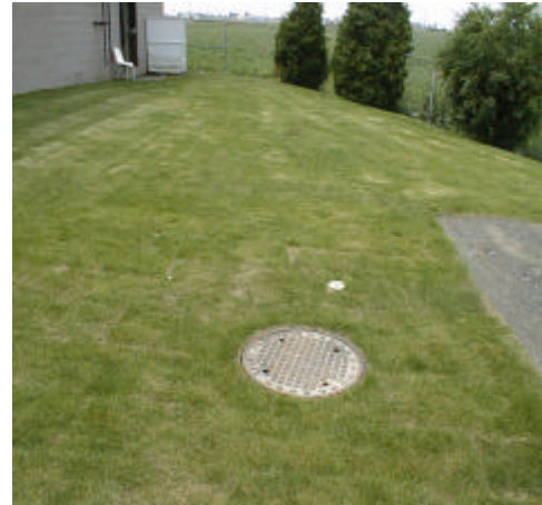
Figure 3 Two transformers connected back-to-back, one directly buried in the ground and the other in a standard sewage pipe. The transformers are presently energized at full load.
