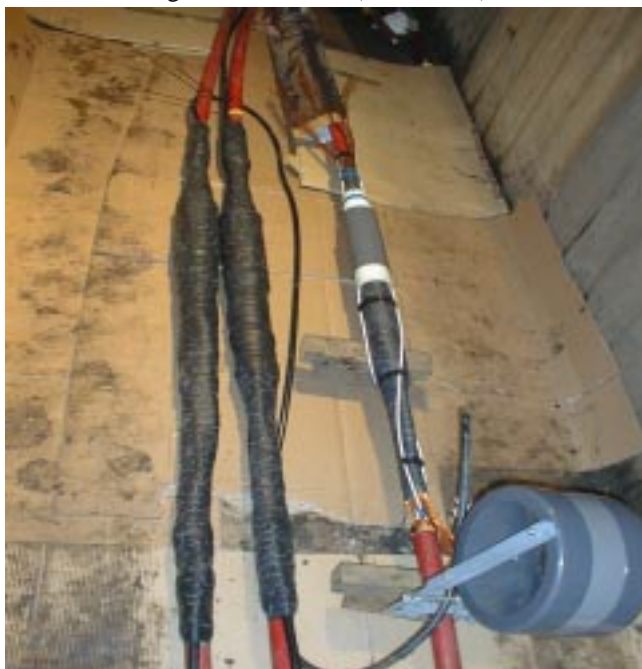
Figure 2: Three electrical / optical joints, made by TKF. The two white strings in the right joint contain the glass fibres, and lead to the white / grey organiser.
