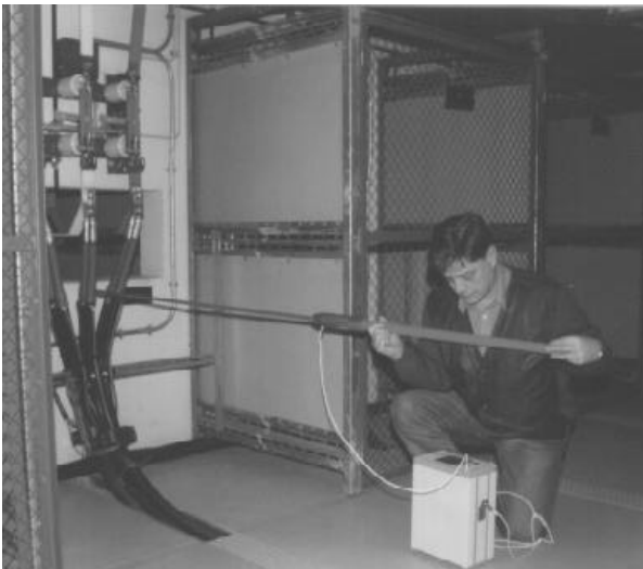
Figure 2: Portable instrument (AIA) and wave-guide probe used on a XLPE termination.
