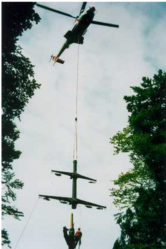
Photo N°4 : Placing in position the top element of the prestressed concrete pole assembled by helicopter in July 1996.
