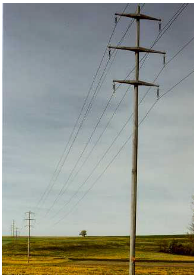
Photo N°1 : Typical concrete pole on a 60 kV line in Switzerland
