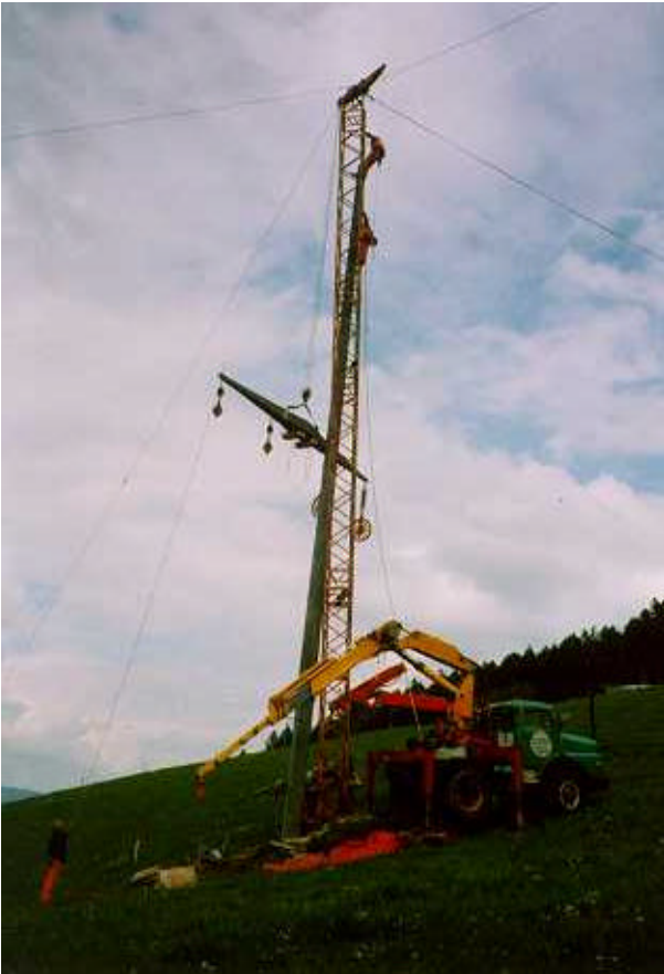
Photo N°2 : Placing in position a bracket of a 60 kV concrete pole with a braced formwork assembly combined with a tractor borne winch
