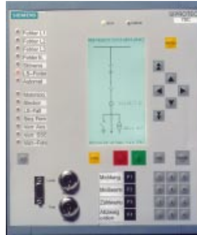
Fig. 4 : New Protection Metering and Control Device
