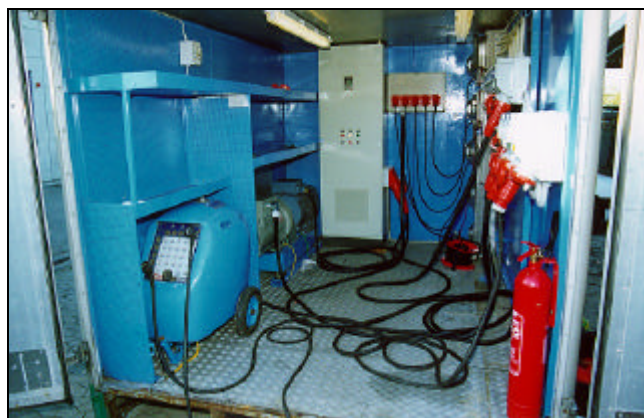
Figure 1 Interior of NESAs movable low voltage load. In the background is seen the VLT with motor and generator. In the foreground is seen a 35 kVA arc welding unit.
