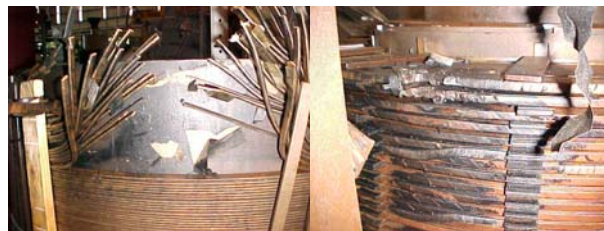
Figure 4: damages in the tap coil (left) and HV winding (right). Relatively low damages were due to the fast trip of the transformer differential protection.
