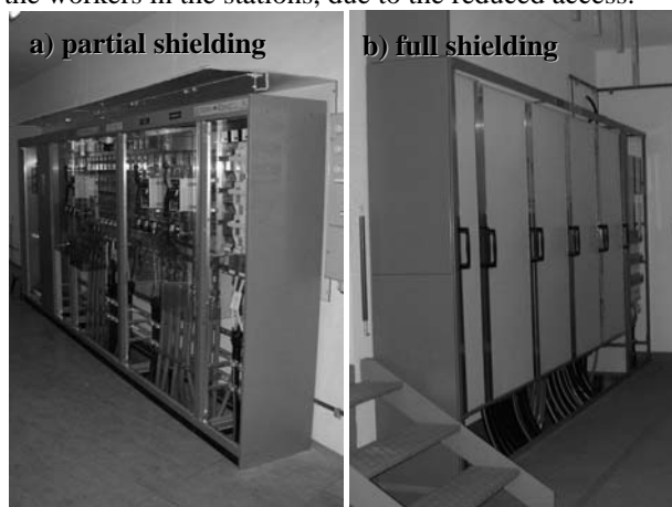
Figure 8: LV distribution board with partial and full shielding.
