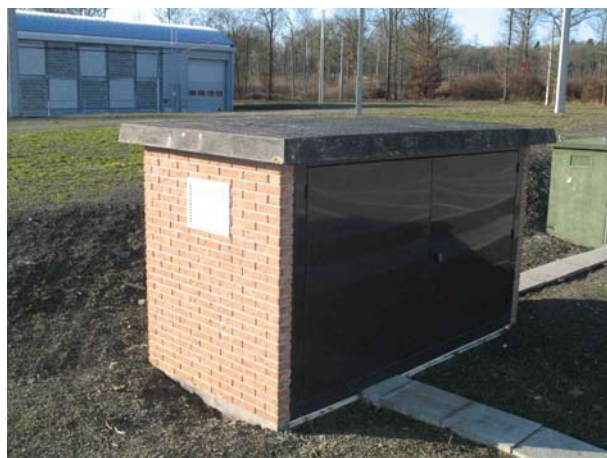
Prefabricated substation in the winter sunlight
