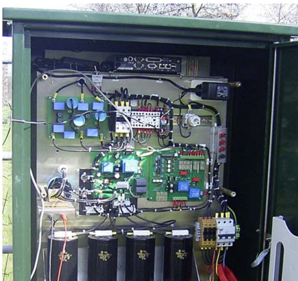
Figure 3. Close-up of the PQO cabinet.
