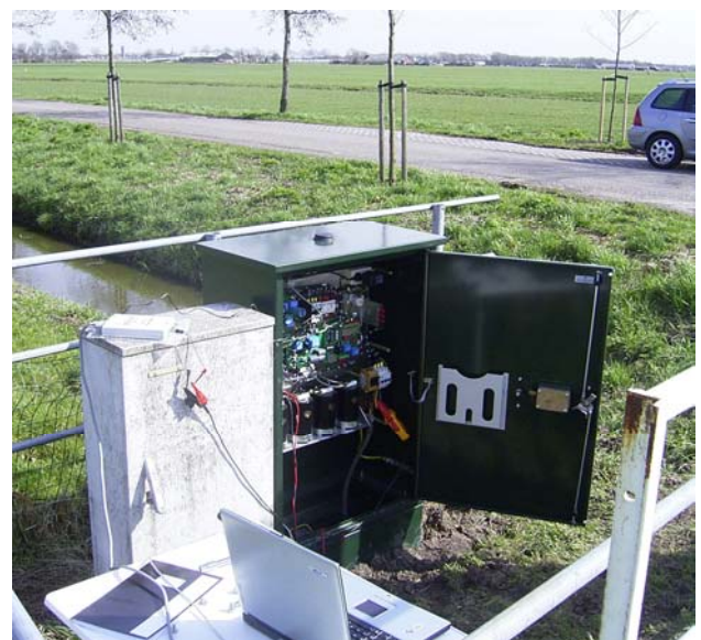
Figure 4. PQO cabinet next to the customer's interconnection box.
