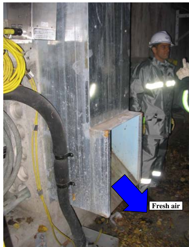
Figure - 5: Upgraded existing vault: central chimney for incoming cold air
