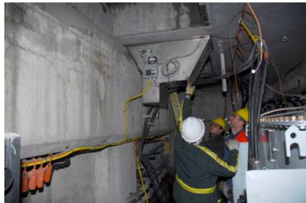
Figure - 6: The blower box at the center of the vault pushing in the incoming fresh air
