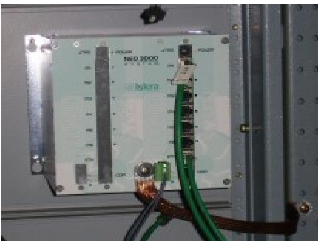
Figure 7: Dedicated CPU installed in substation Črnuče
