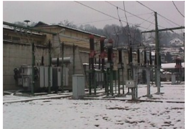
Figure 4: Substation Črnuče in Ljubljana
