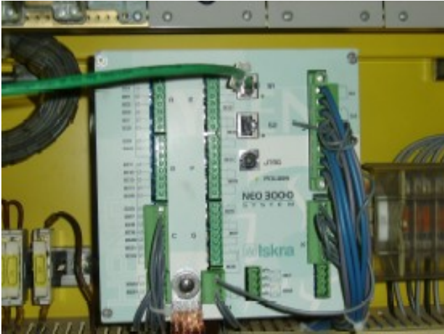
Figure 6: Dislocated I/O unit installed in the substation Črnuče.
