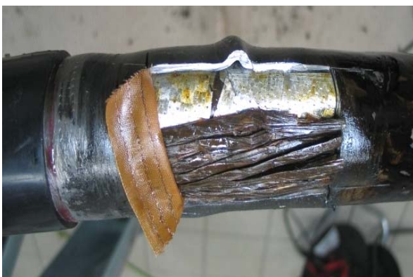
Figure 8: Mechanical damage due to strong bending causes PD in PILC insulation
