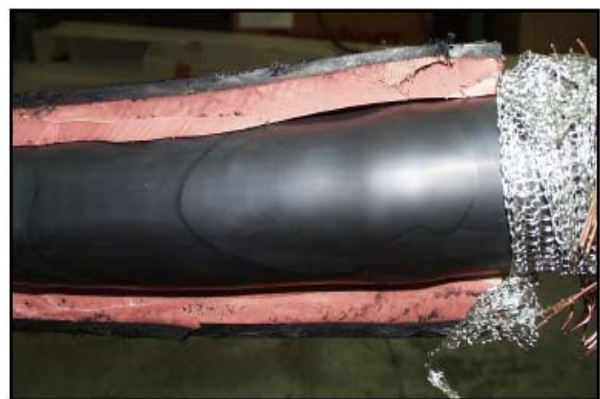
Figure 10: Gap between field stress tube and insulation tube due to incomplete shrinking
