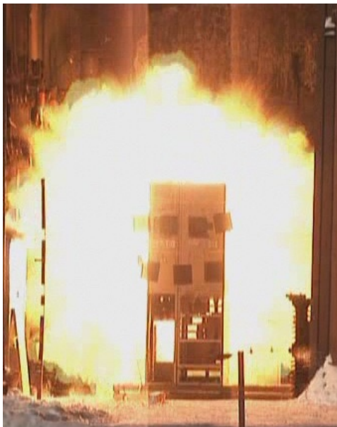
Figure 4. ETALON switching panel tested by 31.5kA internal arc initiated in busbar compartment. Front view. (Photographer Alexey Pasko)
