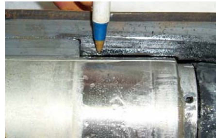
Figure 3. Dissection of a type A joint. The inner Al sleeve is sometimes not connected to the cable connector, which is at high voltage. Note also that the inner semi-conducting material (at the tip of the pen) is not in close contact with the sleeve. Dielectric breakdown occurred through the insulation, to the left of the pen.
