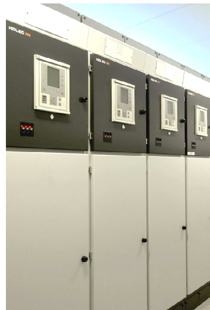
Fig. 5 Example of MV switchgear installation in Finland
