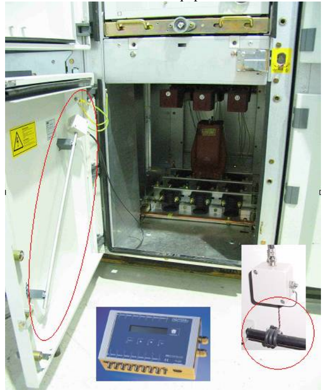
Fig 5. IPD system, antenna and Rogowski installation detail
