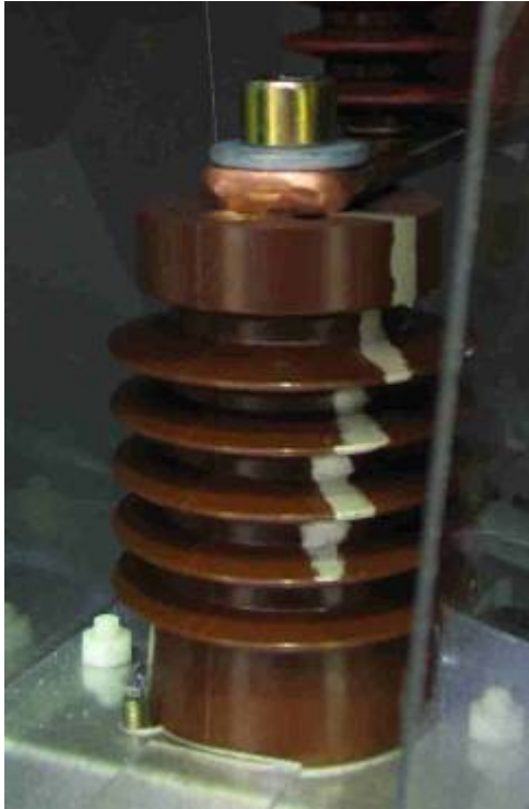
Fig 2. "Low" post insulator with conductive HV defect
