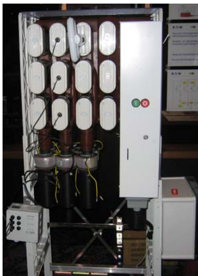
Figure 5: Magnefix with short circuit indicators, current transformers and mobile network connection
