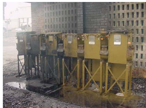
Photo 1 – Oil switchgear failure due to an internal arc
