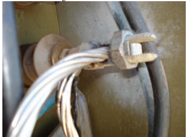
Figure 5: Neutral Failure on transformer bushing
