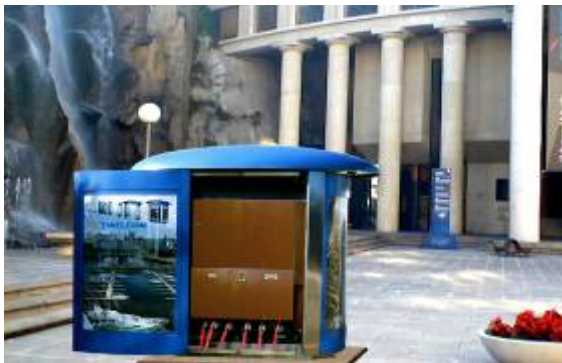
Image 4: Pad mounted substation concealed by a CeTur enclosure.
