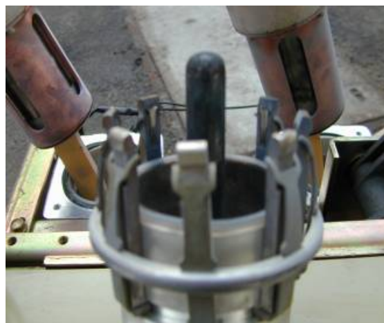
Fig.10 - Phase S fixed contact: note the arcing contact (stood) and t the circular main contact around it -
