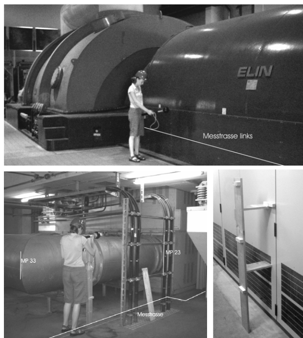
Figure 4: left: 170 MVA generator and 7 kA line coated with iron pipes. Right: probe-positioner
