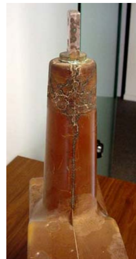
Traces of tree structure on a current transformer
