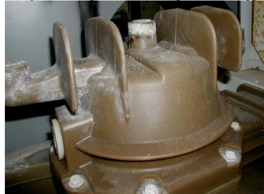
Traces of chalking on an insulating bulb
