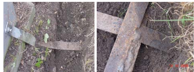
Figure 4. Degradation by corrosion of horizontal electrodes installed in 2001
