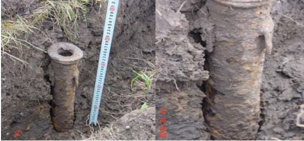
Figure 2. Corroded elements of the earthing system installed in 1965 to Cluj HV/MV substation
