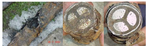
Figure 1. Degradation and electric failure of a underground three-phase cable due to the corrosion of the metallic shield made of steel strips
