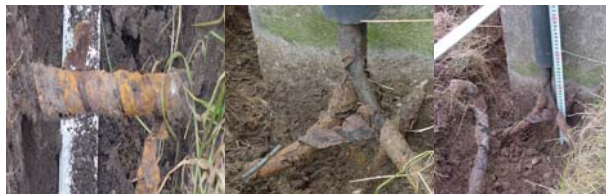
Figure 3. Corroded armors of control and signal cables
