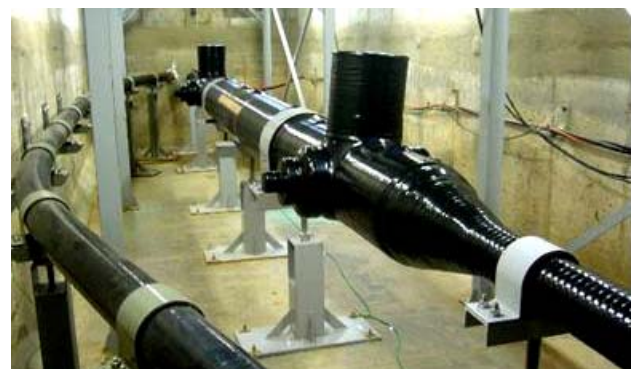
Figure 7 HTS Joint in Underground Vault
