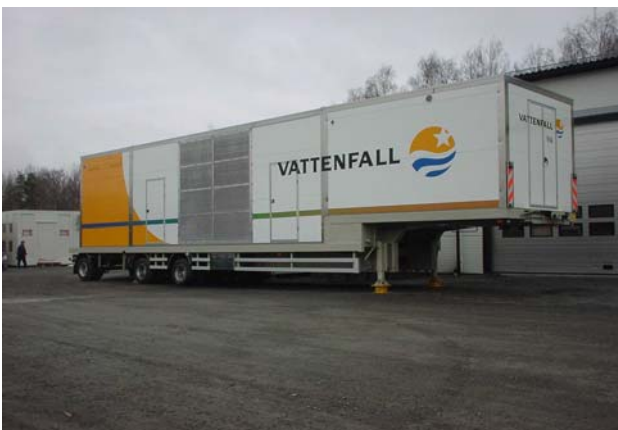
Figure 1 52/24(12) kV mobile substation
