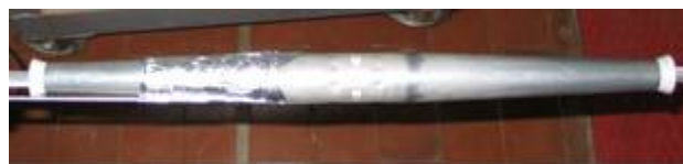
Fig. 8: Photograph, joint, Type 3
