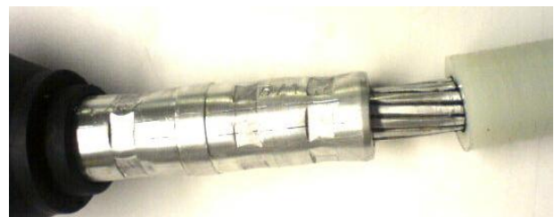
Fig. 5: Incorrect mounted joint
