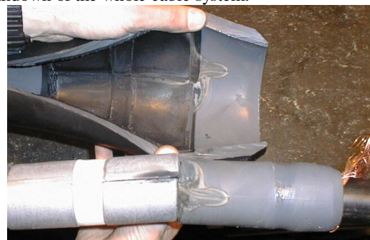
Fig. 11: PD activity due to improper bending of joint
