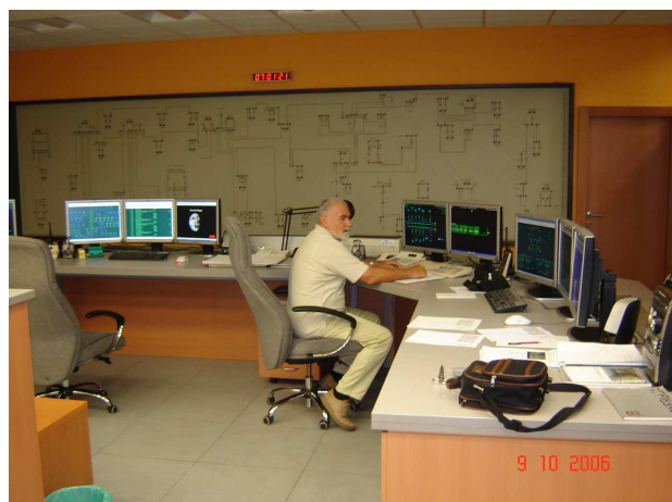
Figure 3: Operator workplaces in control centre Rijeka
