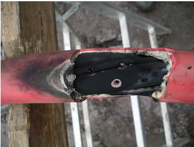
FIGURE 9: Stope cable after earth fault triggered by nail
