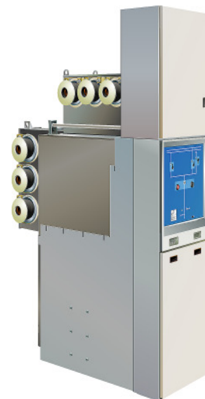
Fig.3: Gas insulated switchgear GHA, 40.5 kV, 2500 A, 40 kA 3 s, Double busbar with B-Link sleeves
