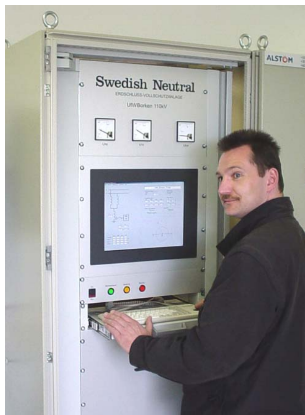
Figure 1: RCC Ground Fault Neutralizer, 110kV railway transmission system (courtesy Deutsche Bahn).
