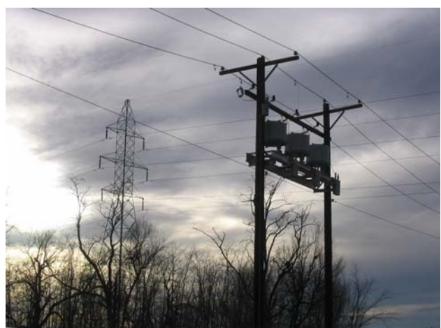
Figure 10. 1200 kvar filter bank installed near the sensitive customer for power factor correction and harmonic control.
