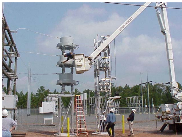
Figure 4. Tuned capacitor bank at the substation to control harmonic levels.
