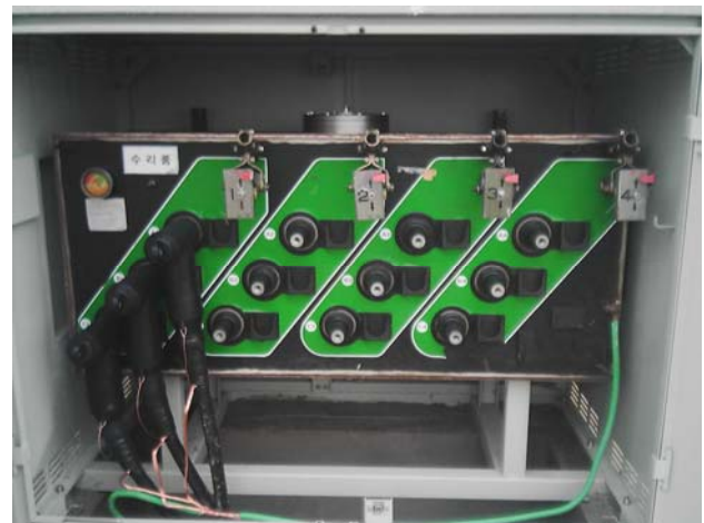
Fig. 1. A photo of SF 6 MV switchgear
