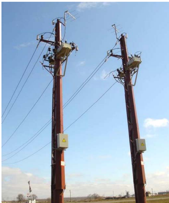
Figure 3 – Application of the Tavrida Electric reclosers in the gas-and-oil producing industry
