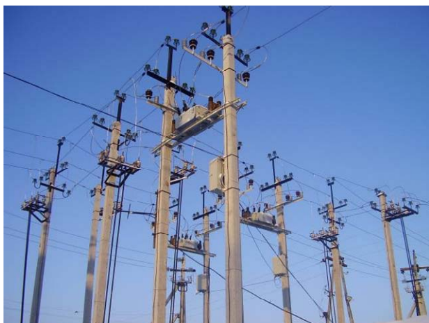
Figure 5 – Substation application of the reclosers in Siberia
