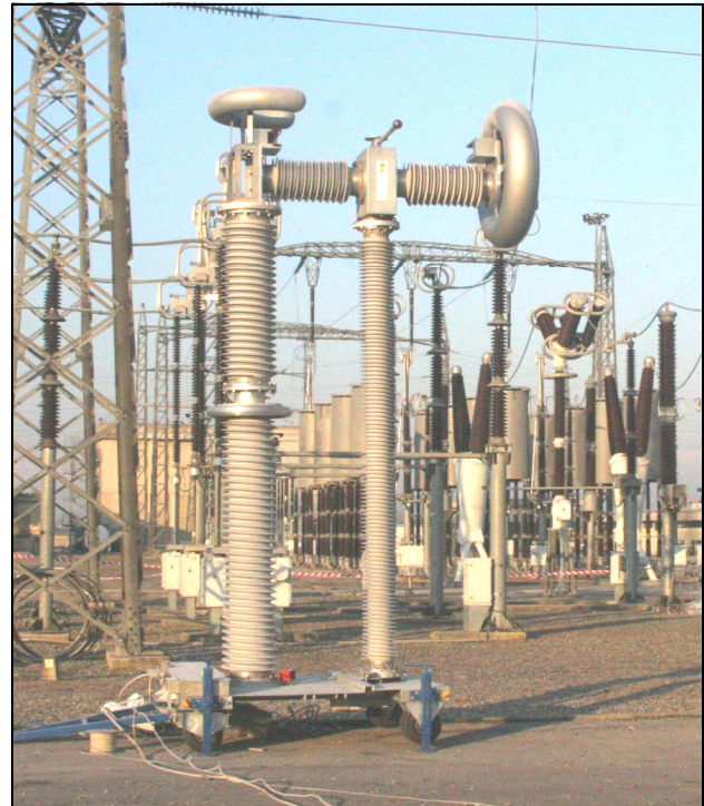
Figure 4 – The voltage divider: 400 kV configuration
