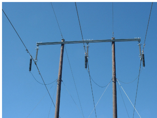
Fig. 5. A picture of the new 130 kV transmission line between Orrby and Station A.
