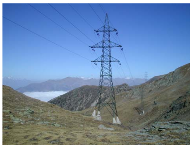
Figure 1: 110kV overhead line in a high alpine region
