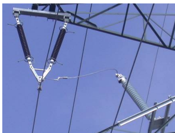
Figure 5: Line arrester application on the 110kV steel tower
