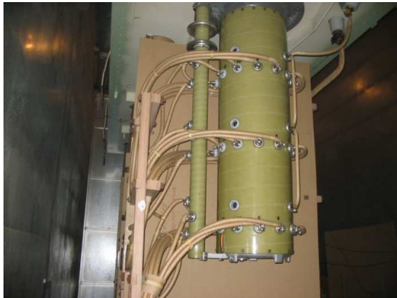
Fig. 2 - Power transformer with vacuum diverter switch OLTC
