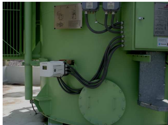
Fig. 4 - Power transformer oil on-line monitoring.
