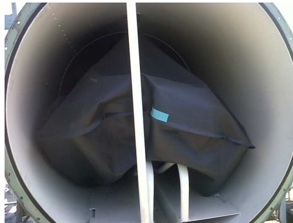
Fig. 3 - Auxiliary tank with bladder separator.
