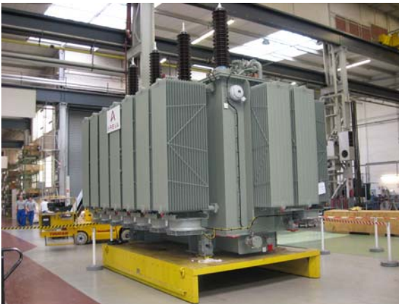
Fig 4: First 40/50 MVA, ONAN/ONAF grid coupling transformer with new speed controllable fans with EC technology manufactured in Germany in 2009
