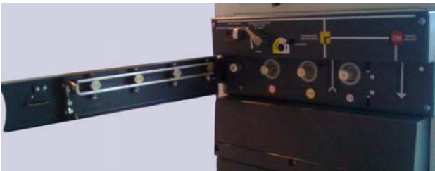
Fig 1: example of dedicated access for cable test purpose
