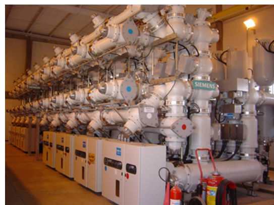
Figure 2 – Anhanguera GIS 345/230/88 kV Substation
