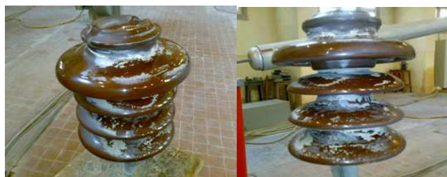
Fig.(1). Polluted Insulators
