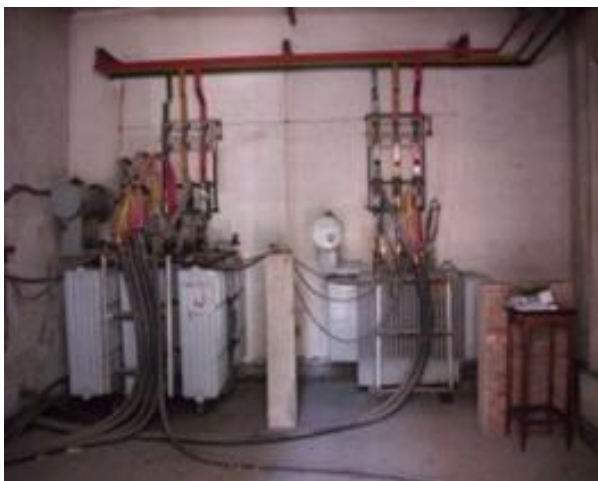
Fig.7. Magnetic field measurement at distribution substation
