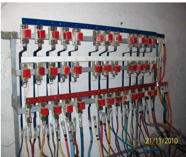
Fig.1. Low voltage panel
