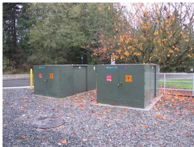
Figure 3 Loop Tap Switches on Site
