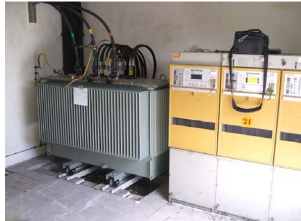
AMDT 400 kVA at ERDF Tisans Substation, near Paris.
