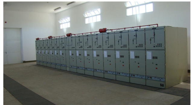
Fig. 1 view of 13, 2 kV Indoor Single busbar metal-enclosed switchgears.
