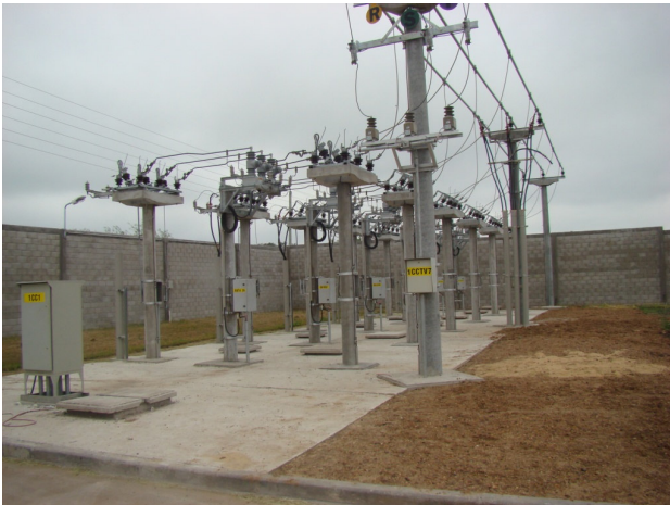
Fig. 2 view of 13, 2 kV Outdoor Single busbar with automatic reclosers.
